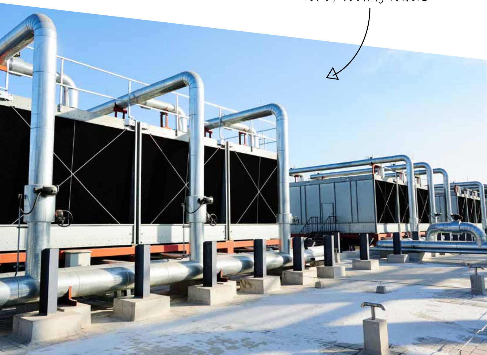
Set of cooling towers
